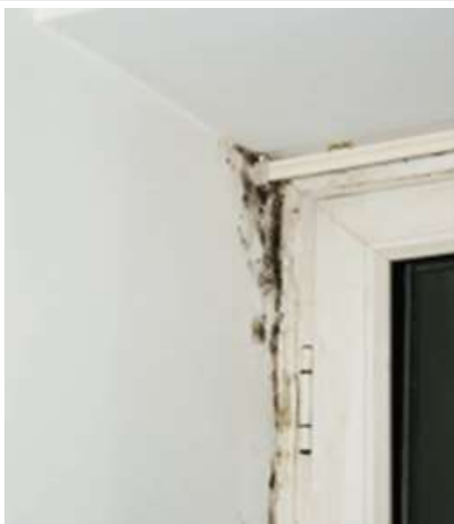
Figure 1.1 Mildew caused by condensation of thermal bridge
